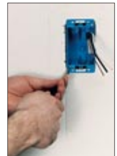
Secure Box in Wall
