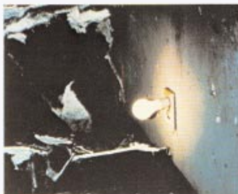
⑥ This receptacle is located in room 206 and is operative after flashover. Room temperatures during flashover shown in Graph B. See Diagram II.
