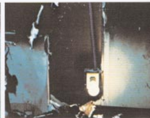
⑦ This photo shows same receptacle as photo #6, but the wall board was removed to show wiring and box intact. See Diagram II.
