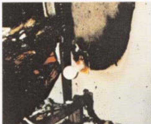
① This wall receptacle in the apartment master bedroom shows the extent of fire damage to bed frame, wall and outlet plate, while circuit operation is demonstrated by light. Recorded room temperatures are shown in Graph A. See Diagram II.
