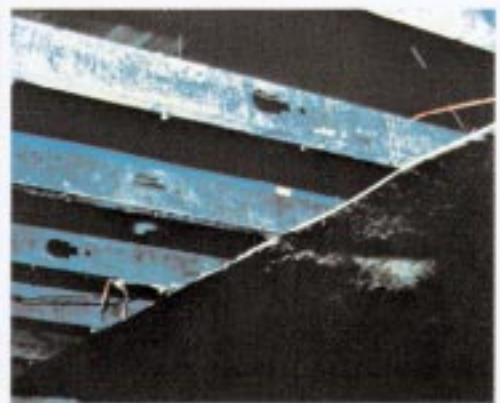
5 The raceway in this photo is mounted above room 206. This room was one picked for a flashover fire on final day. See Diagram II and Graph B.
